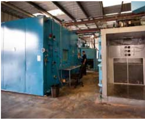
Large Array of Temperature, Altitude and Humidity Testing Chambers
